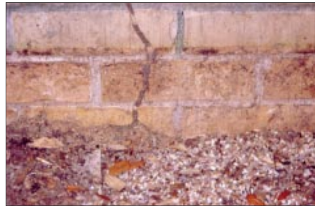
Termite shelter tubes on foundation wall.
