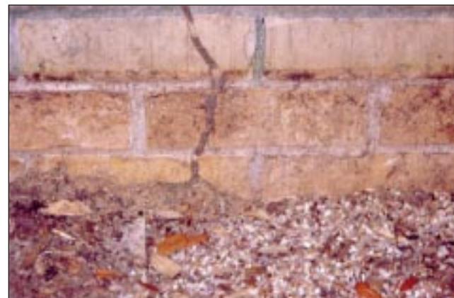
Termite shelter tubes on foundation wall.
