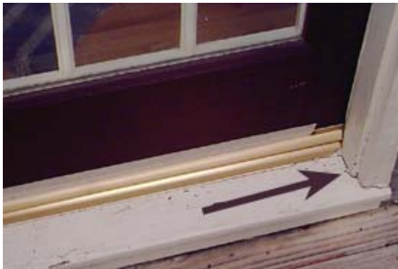
Rain can seep into unprotected wood in doorframes.
