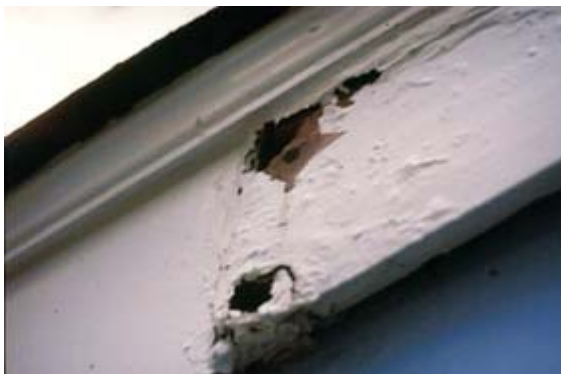
Water-damaged fascia can lead to termite problems.
