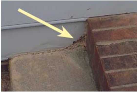
Water splashing on porch steps can lead to decayed siding.
